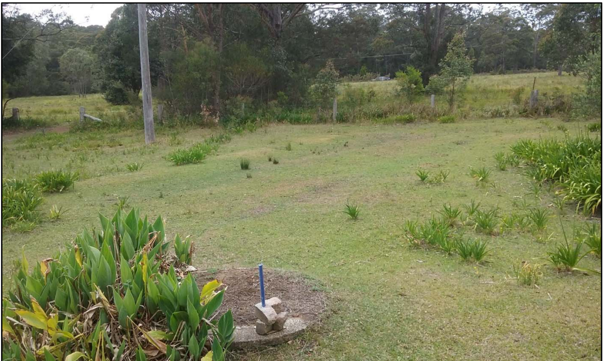
Plate 3: Septic tank and trenches.
